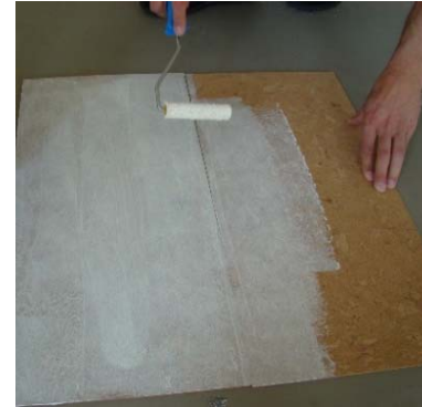
3. Apply a thin layer of adhesive to the back side of the cork. Ensure full coverage but avoid adhesive puddles.
